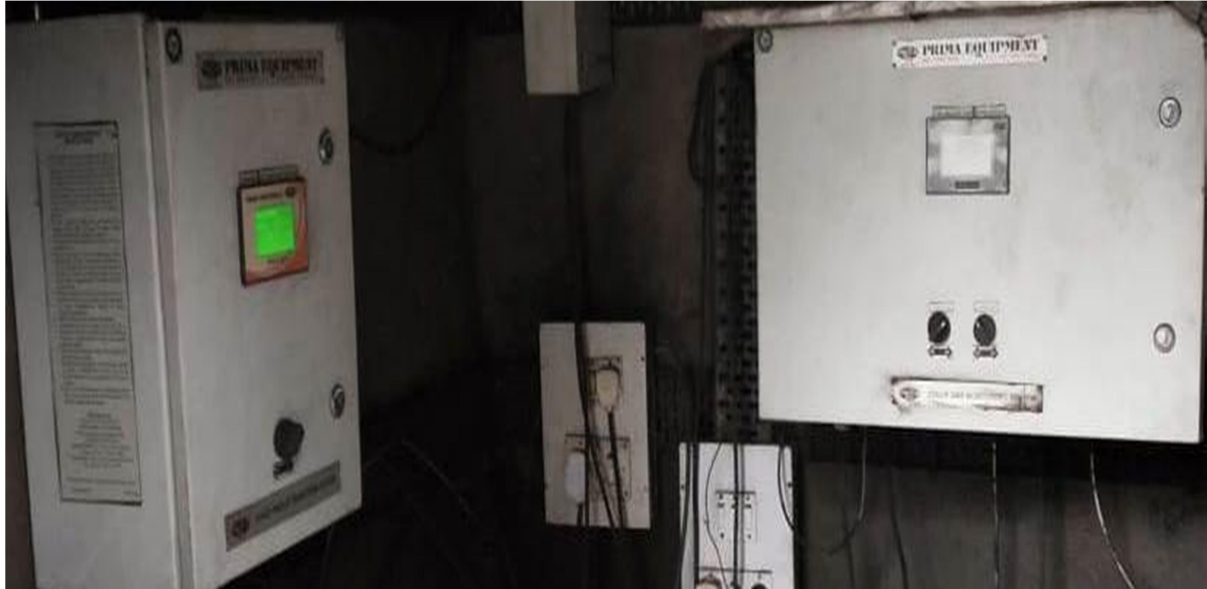
Stack -1 Online Continuous Emission Monitoring System (CEMS)
