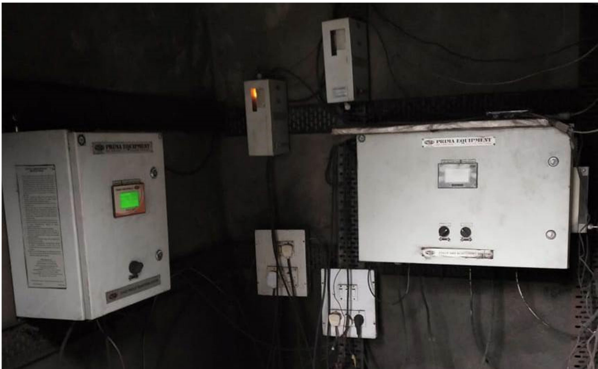
Stack -2 Online Continuous Emission Monitoring System (CEMS)
